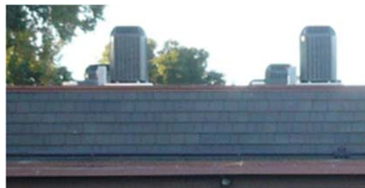
New condensers on roof of Gunn Buildings
