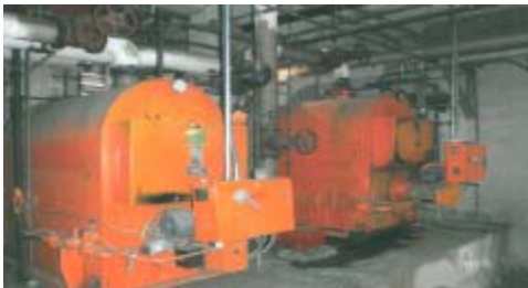
Boiler Replacement - Before
